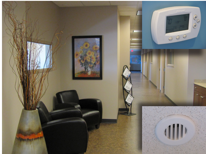
New office space with individual thermostats and dampered outlets
