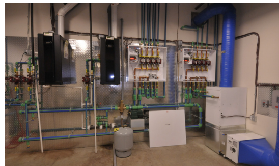
Mechanical Room featuring Hi-Velocity System Products
