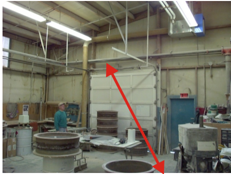
Drilled outlets to provide air curtain around shipping door....
